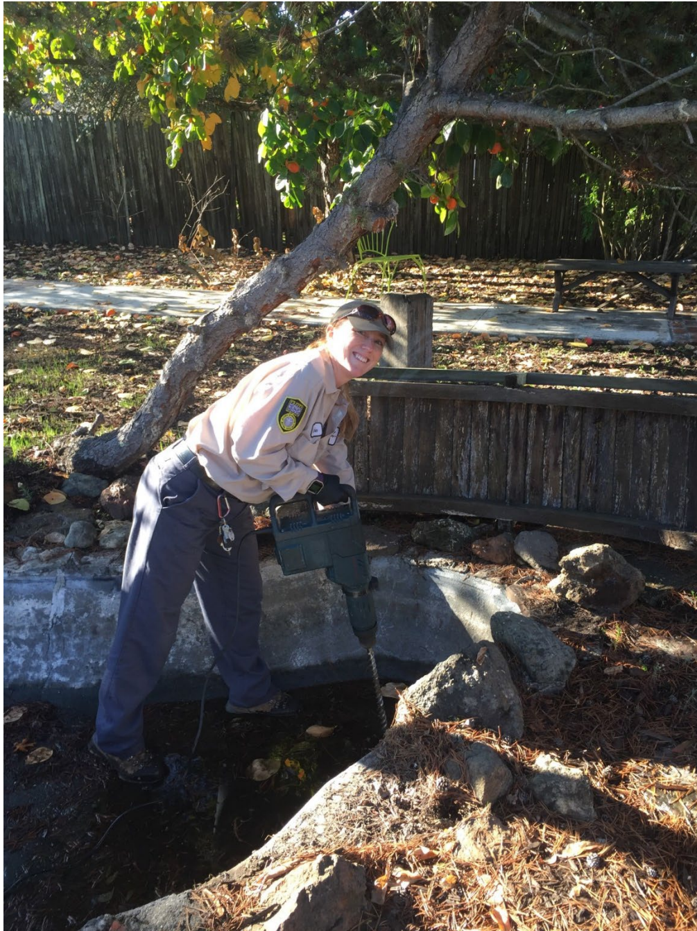
Figure 6- Vector Control Technician Stephanie Busam is drilling holes in a pond so it will no longer hold water. This is a source reduction program offered to property owners to help eliminate mosquito breeding habitats.
